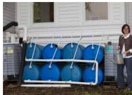
Rain barrels provide a sustainable source of water for keeping the Arts Center's gardens flourishing. Photo by Natalie Jeanne Photography
